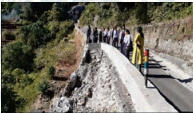
Field survey on Measurement and monitoring of Landslide at Shiv Khola basin, along the Hill Cart Road, on 25 th November, 2022, at Rongtong, Tindraria area in Darjeeling Himalaya
